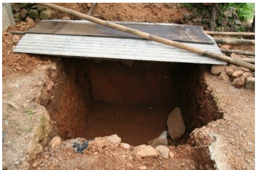
Figure 7. Septic tank being built next to a house in Phaniewlah. Walls are left permeable, which is likely to be the main agent of water contamination.
