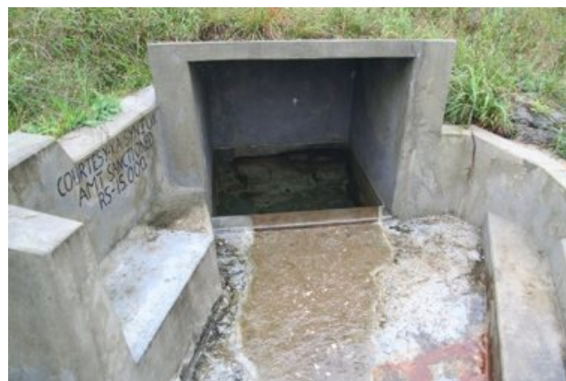
Figure 4. Example of one of 28 water spring constructions that were financed and developed by the project in 2015-16 under the community micro-project scheme. Samples of water are annually analysed.
