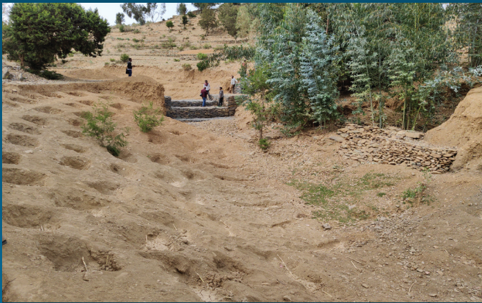
Revegetating gullies to reduce soil erosion, with a gabion check dam in the distance.
